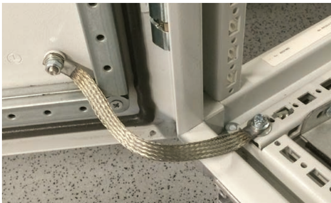
Figure 12 – nVent ERIFLEX MBJ used for equipotential bonding according to NEC and UL508A
