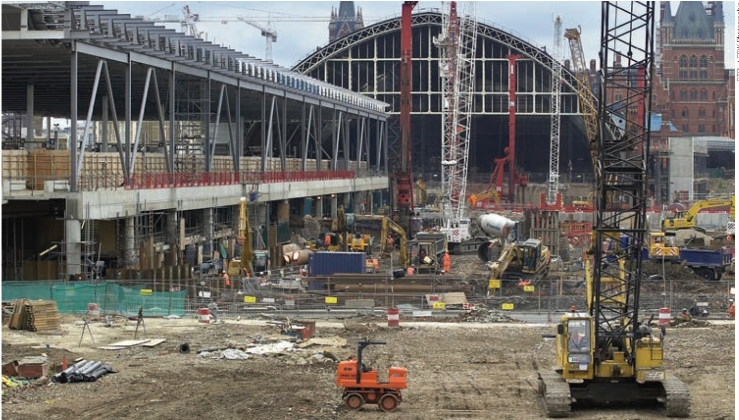
View looking toward the St. Pancras Station shows work on the Thameslink Box and half the deck extension.
