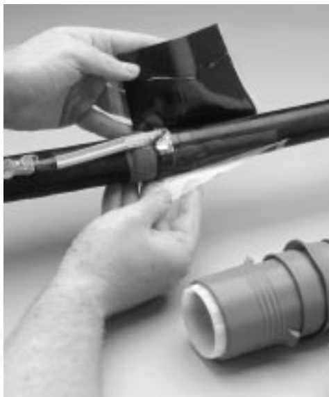
Photo 6: Applying the stress control patch. In line with initial outer layer cut and over the bonding braid.
